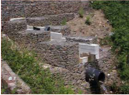
Prosser Terrace, Abercregan, Land Drainage/Highway Drainage Scheme Gabion works at surface water outfall
